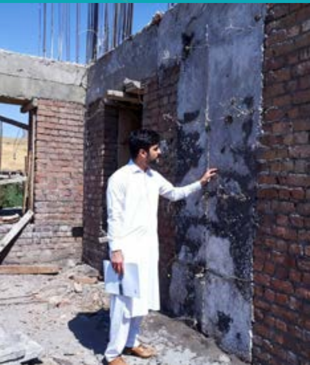
Figure 1. Identifying segregation issues in building work
